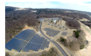
Iwaki Solar Power Plant
