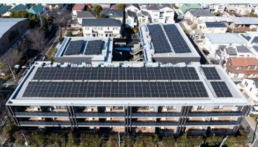
Solar panels installed across the entire rooftop
