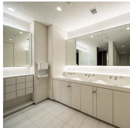
Installation of a Compartment in the Powder Corner of the Restroom with a Refreshing White Tone
